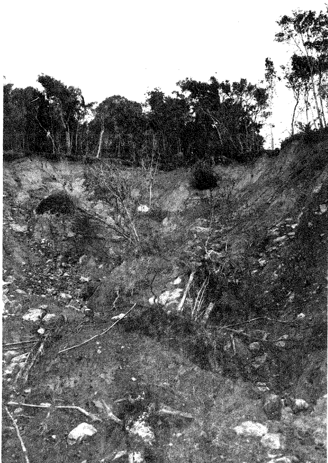
Severe damage due to a landslide after a period of heavy rain, Puerto Rico.
