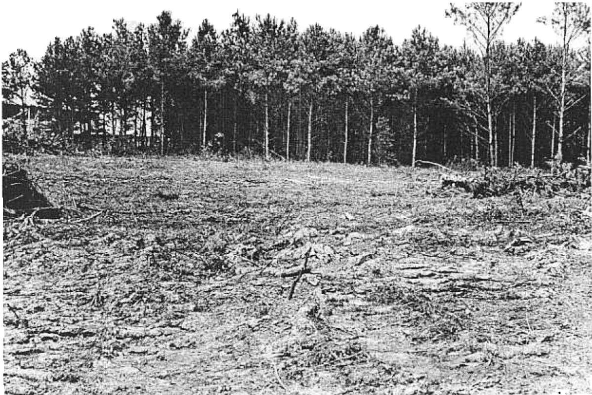
Figure 7. — After extraction of all trees, the Cedartown site was free of stumps and debris. Skidder action has filled in most of the stump holes.
