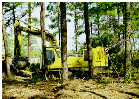
Costs of Mechanical Fuel Reduction Treatments, Fig. 3 Boom-mounted mastication machine processing midstory vegetation in a wildland urban interface near Havelock, North Carolina, USA
