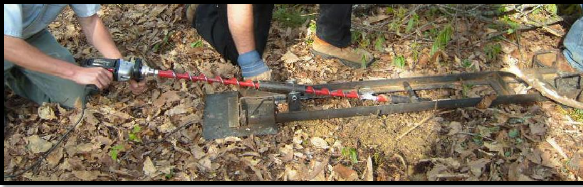
Figure 3. Auger and jig setup used to install bulb and hose at known depth and location.
